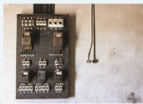
Electrical Switchboard Panels
